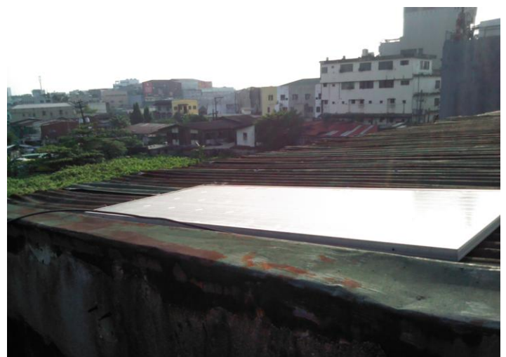
Fig. 6. Photovoltaic module installed on roof top during system test.
